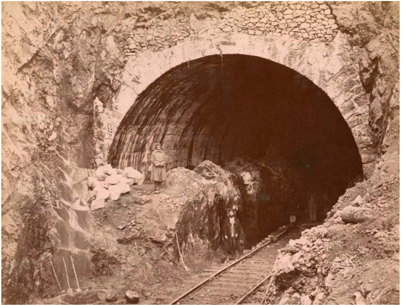
The Surami tunnel under construction. The tunnel (completed in 1890) was a tremendous improvement, not only for oil transport between the Caspian and Black Seas but also for Baku oil, opening a volume gateway to Europe. Source: National Archives of Georgia.
